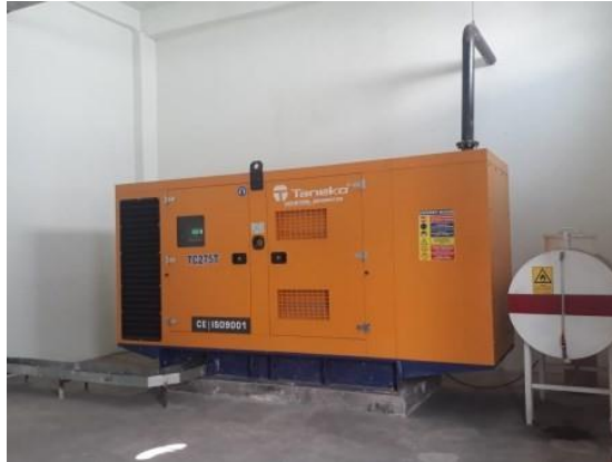
Gambar 2.9 Genset RSUD Cipayung
