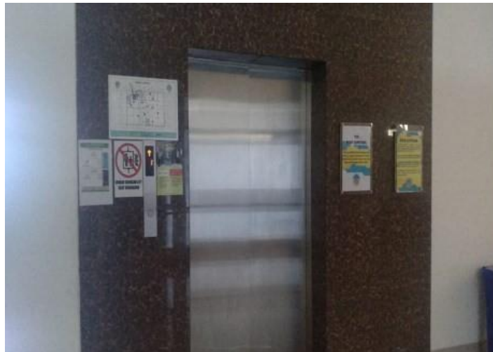
Gambar 2 Lift Gedung RSUD Cipayung
