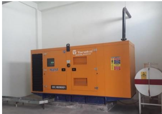
Gambar 3 Genset RSUD Cipayung
